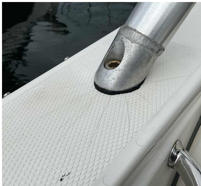
L15. Spider cracking surrounding gelcoat to tower
