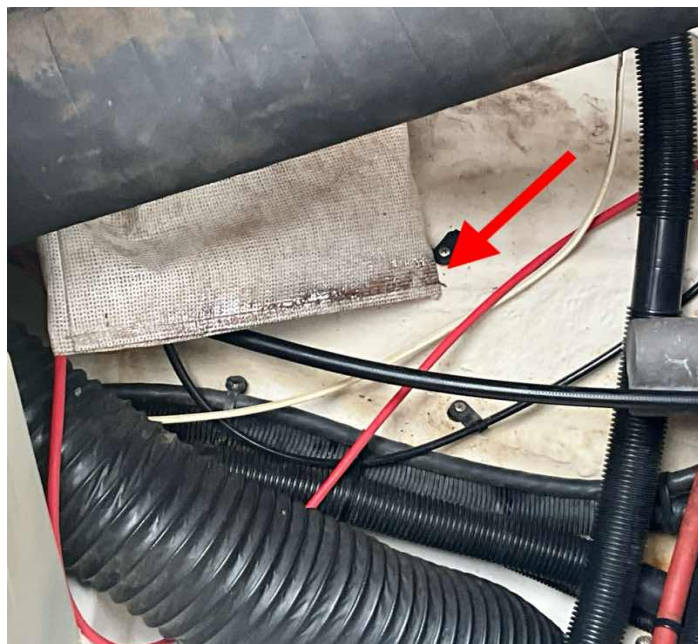
L27. Transom shower leaking
