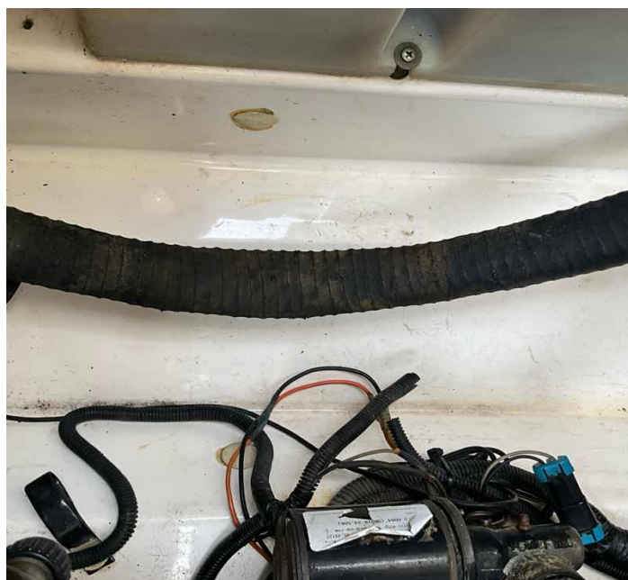
M4. Toilet vacuum hose perished
